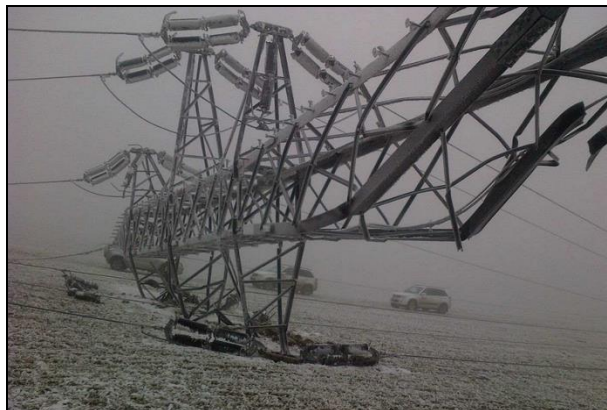
Figure 4. High-voltage masts collapsed due to icing
